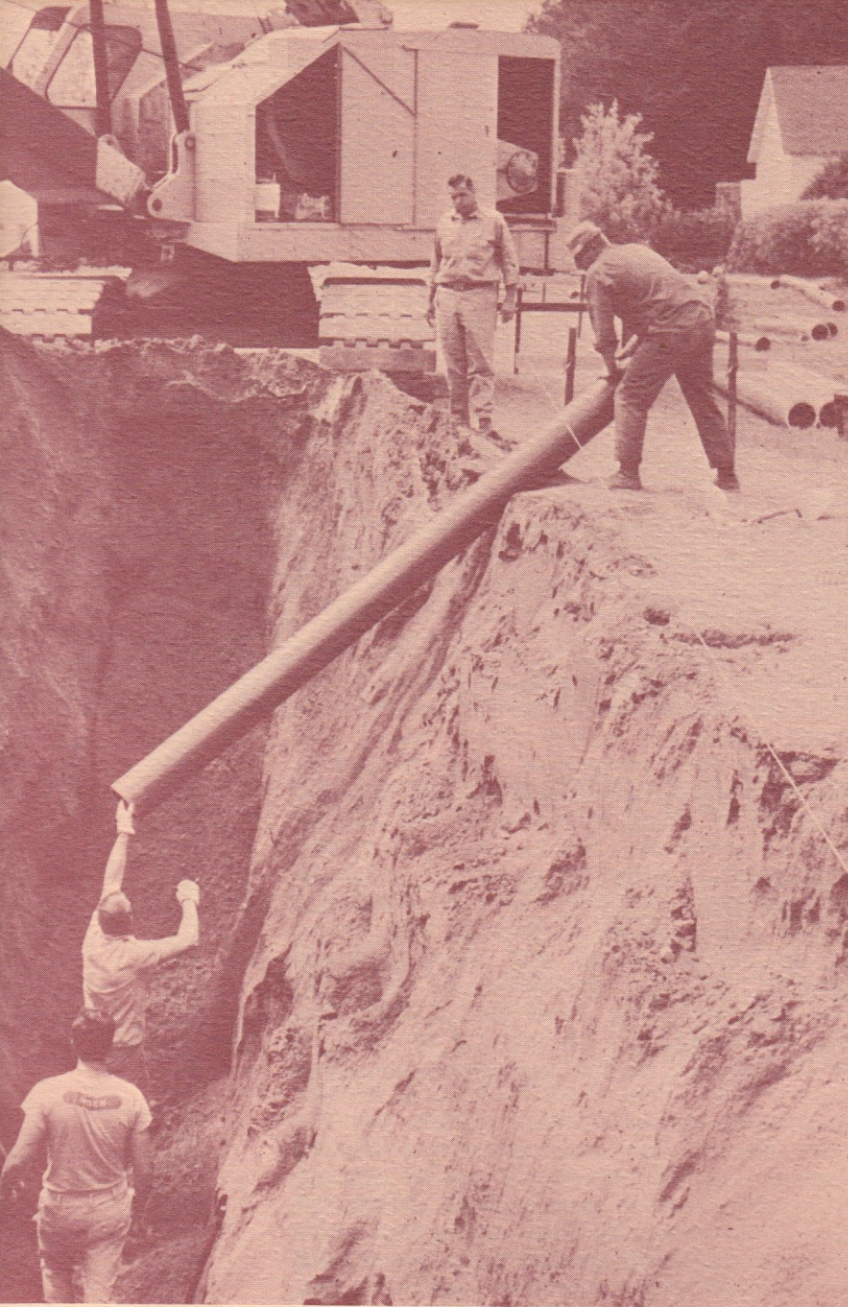
ABOVE: Improvement of Utility Systems will be a High Priority Item During the 1970's.
